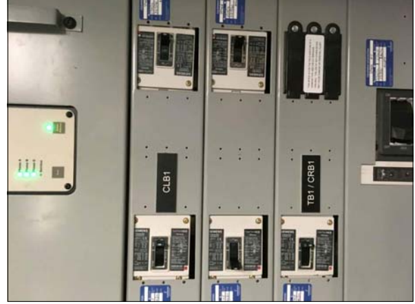
MSBC PANEL INSTALL NEW 50 AMP BREAKER IN THE SPACE SHOWN
